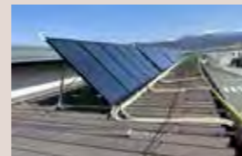
Solar panels installed at Komagane Plant
