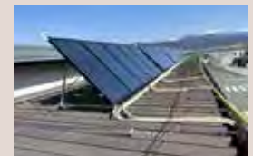
Solar panels installed at Komagane Plant
