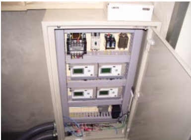
Electricity monitoring systems
