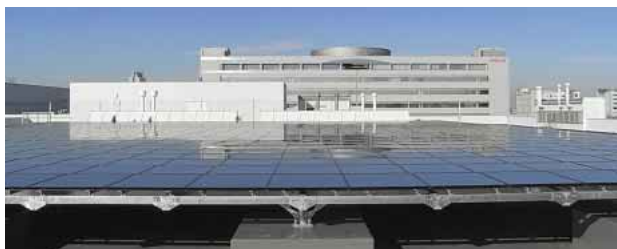
Solar power generator installed on the rooftop of the R&D building
