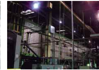
High efficiency illumination that change the plant lights from mercury lamps to fluorescent lamps (NHK of America Suspension Components (NASCO), North America)
