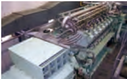
Cogeneration equipment at the Yokohama Office operating since February 2005 (4,450 kW)
