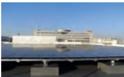
Solar power-generation equipment at the Yokohama Office (100 kW) (In operation since February 2009)
