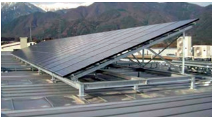
DDS Komagane Plant (20 kW) Commissioned 2008
