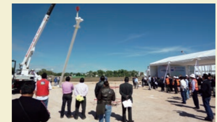
Column erection ceremony held at the time the construction project begins for NHK SPRING MEXICO S.A. DE C.V.
