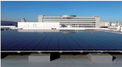
Yokohama Office (100 kW) Commissioned 2009
