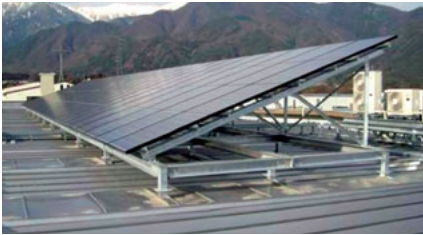
DDS Komagane Plant (20 kW) Commissioned 2008
