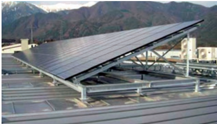
DDS Komagane Plant (20 kW) Commissioned 2008
