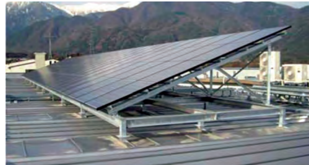
DDS Komagane Plant (20kW, FY2008 operation start)
