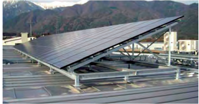
DDS Komagane Plant (20kW, FY2008 operation start)
