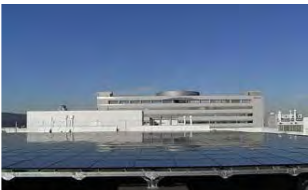
Yokohama Office (100kW, Start from FY2009)
