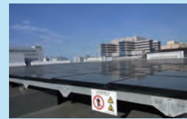
Solar panels installed at our Yokohama Office
