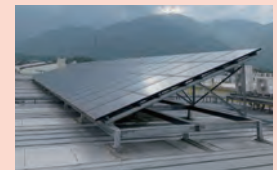
Solar panels installed at Komagane Plant
